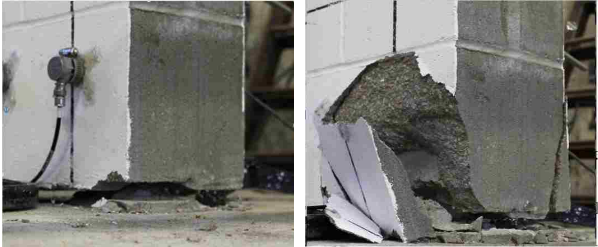
(a) Separation at the Bed Joint
